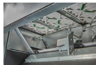
Economizer, Jade Control
